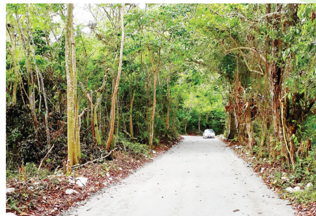
Picture of road resurfaced in Cacoen Castle, Hanover under the Farm Road Rehabilitation Programme
