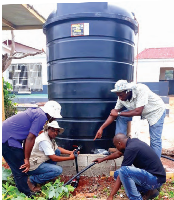
Officers from the On- Farm Water Management Unit installing a rain water harvesting system in Southfield, St. Elizabeth.
